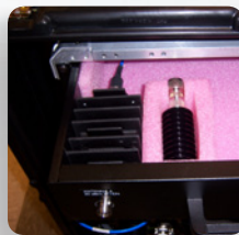
Drawer Containing Antenna A Attenuator
